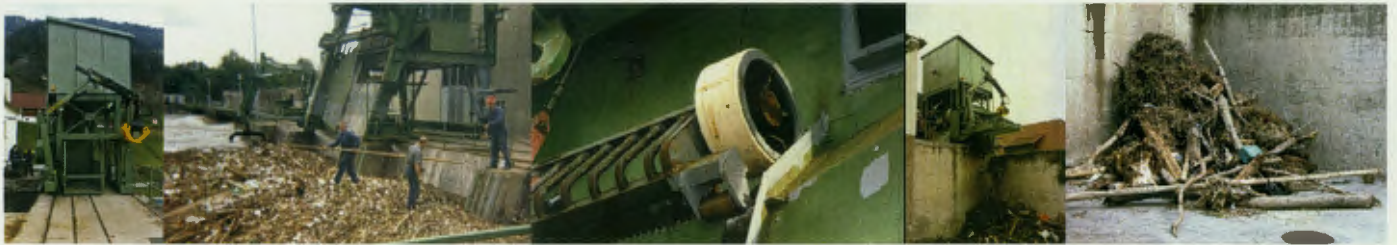
Above, left to right: trashrack cleaner after refurbishment; accumulated debris and driftwood in Gralla; repaired rake at Gralla; debris disposal; debris at St Dionysen
