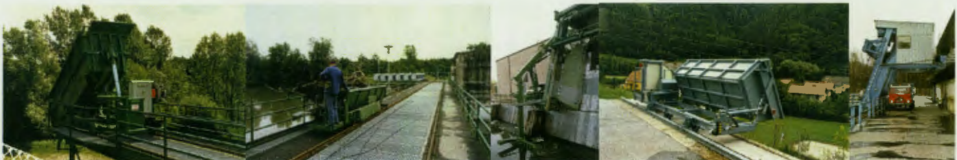
Top, from left to right: Rectangular hollow section as bracket for the crane at Obervogau; hollow section frame at Lauffnitzdorf; the trashrack at Pernegg with crane and container wagon; crane with timber grab at Gralla. Below, left to right: The new container wagon at Gralla; view of the old Gralla wagon; rotating surface rake; new tipped container at Pernegg; the old system at Obervogau
